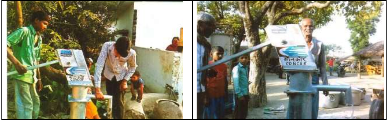
Toilet Blocks in Khatuwas(Raj.) Ghazipur & Handpump at Lakhimpur Khiri (U.P)
